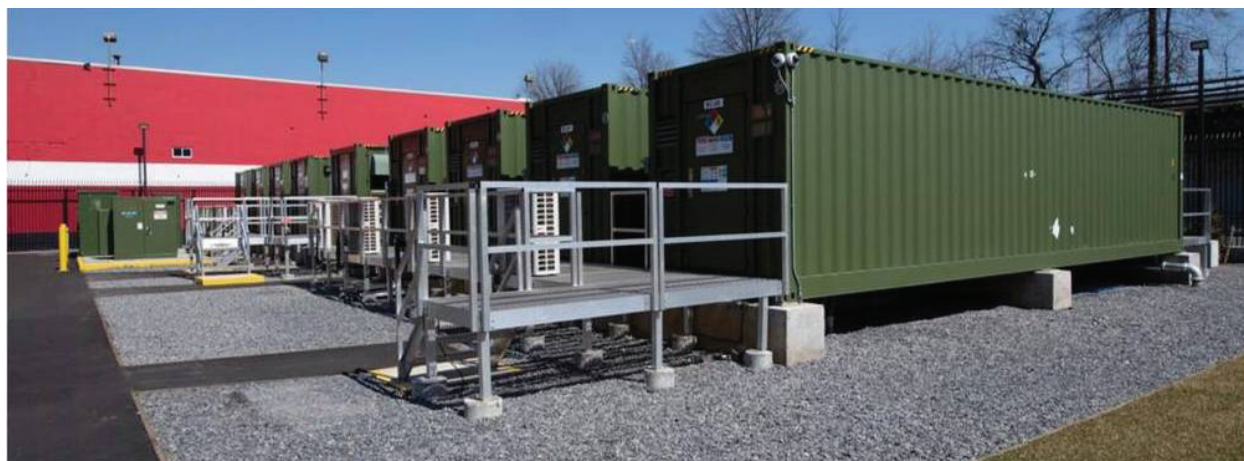
A battery storage facility built to address growing demand in Queens. PHOTO: THE PEAK COALITION
